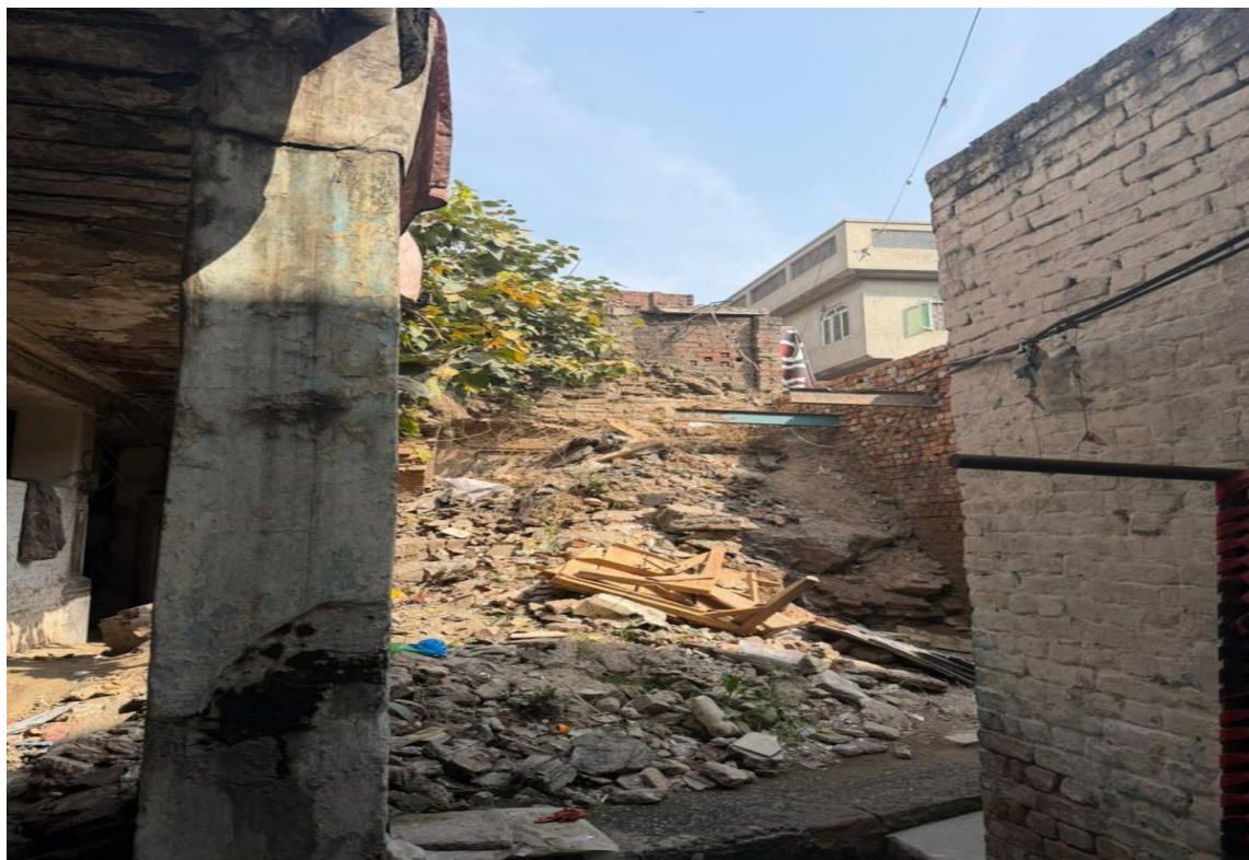
Fig. 7 The crumbling Gurdwara Damdama Sahib (Photo: Madiha Abbas)
