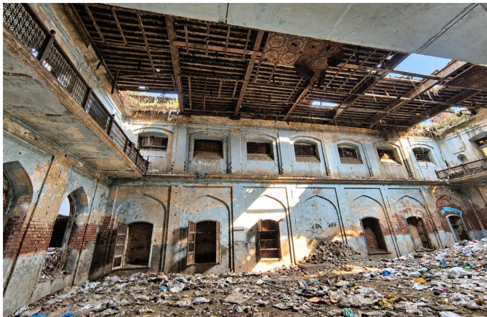
Fig. 15 Gurdwara Sri Guru Singh Sabha, Gujranwala, Deteriorated Interior and Collapsed Roof (Photo: Muhammad Kashif Ali)
